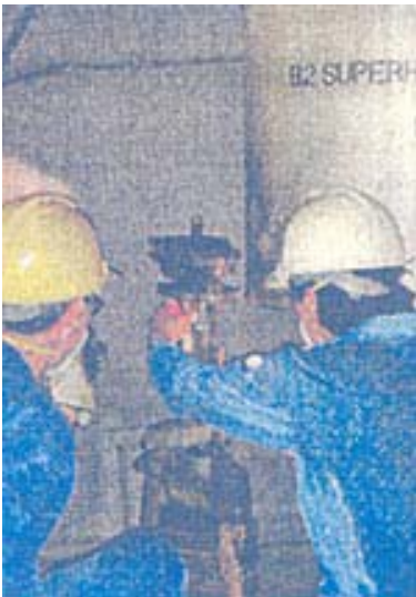
Inspecting a water-tube boiler superheater safety valve.
